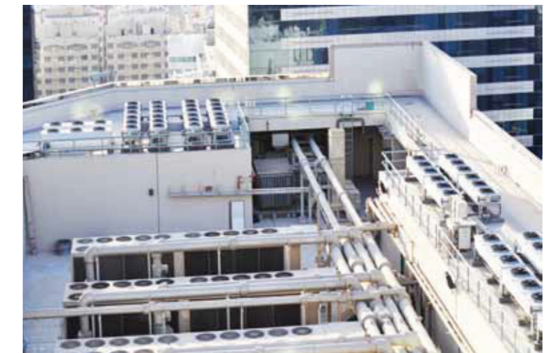
Access to roof mounted HVAC systems can be controlled and unauthorised access easily detected for efficient response
