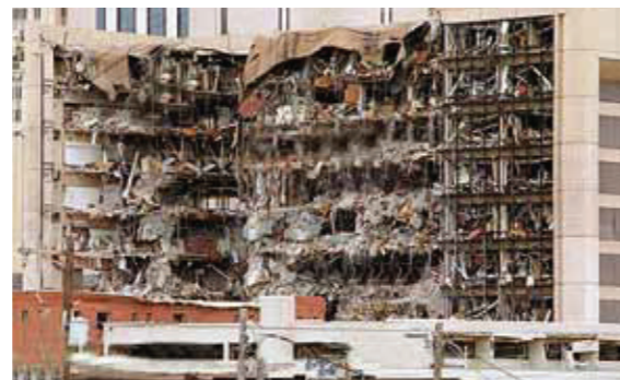
Progressive collapse resulting from a large VBIED, Oklahoma City, USA
