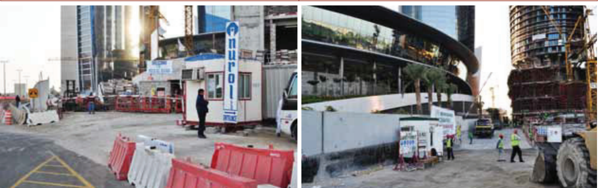
Construction can affect the security of neighbouring occupied buildings
