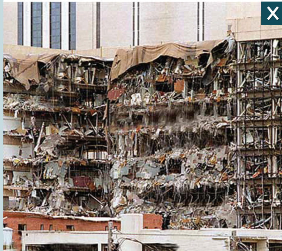
A lack of stand-off contributed to the large number of fatalities and injuries in the Alfred. P. Murrah Federal Building, (Oklahoma City, USA)
