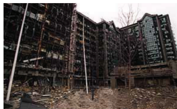
Glazing failure resulting from a large VBIED, Canary Wharf, London, UK
